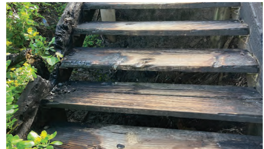
Figure 310: Damaged stairs at Blue Lagoon Beach.
