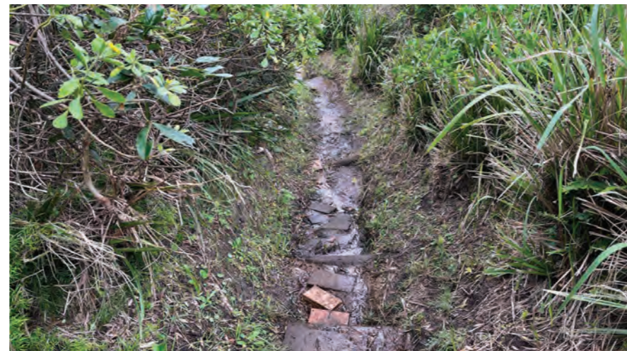
Figure 353: A section of informal access to Jenny Dixon Beach which is unsafe.
