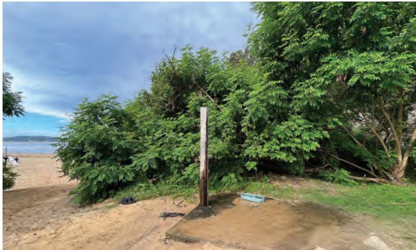
Figure 343: Old shower at Ettalong Creek, south of Umina Beach.
