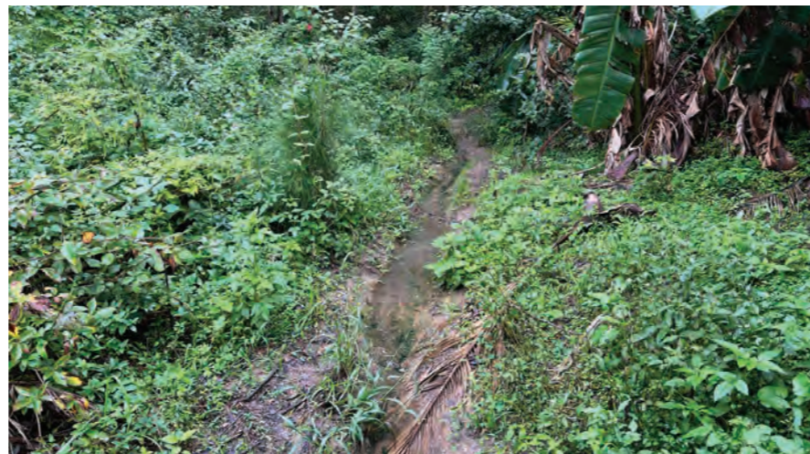
Figure 295: A particularly poor quality section of the Avoca Lake path posing a slip hazard.
