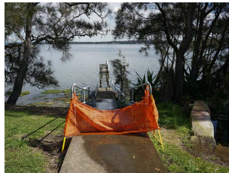
Figure 67: The jetty at Mutumba Road Reserve has seen better days.
