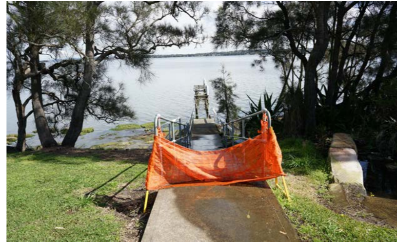
Figure 194: Budgewoi Lake, Mutumba Road Reserve node: facilities there are good but jetty in need of repair.
